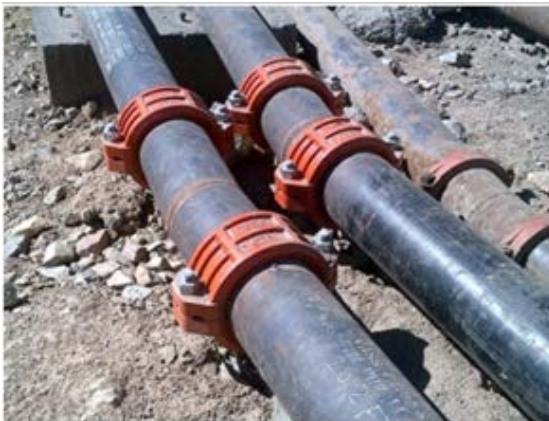
Shurjoint #RX-3000 Ring Joint Couplings used in conjunction with 80 pipes
