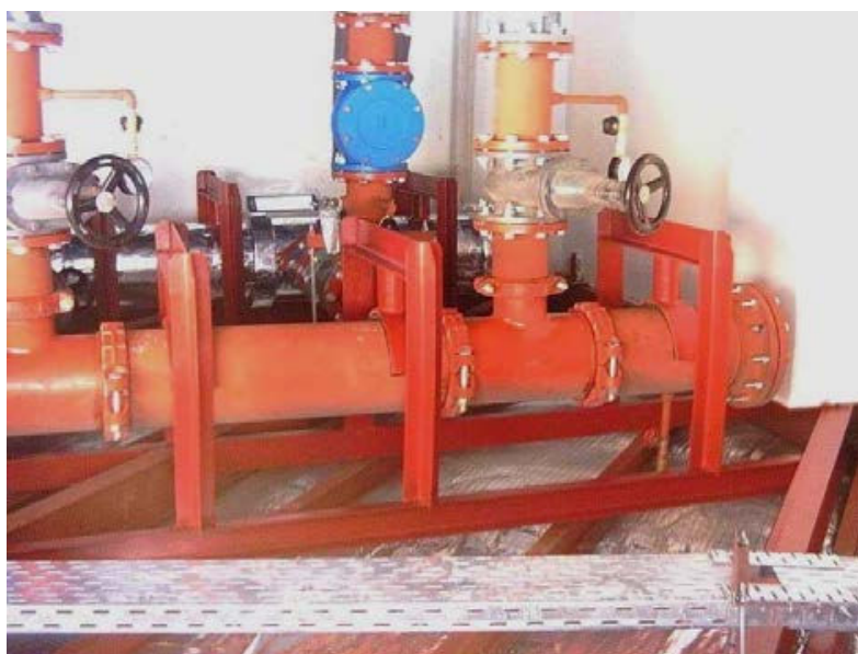
24" Dia Chilled Water Lines inside Pump Room
