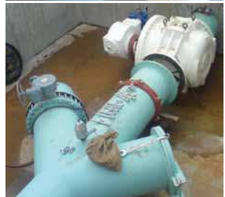
48" (1200mm) Model R-88 couplings used in a water treatment plant, Quarry, Utah, USA
