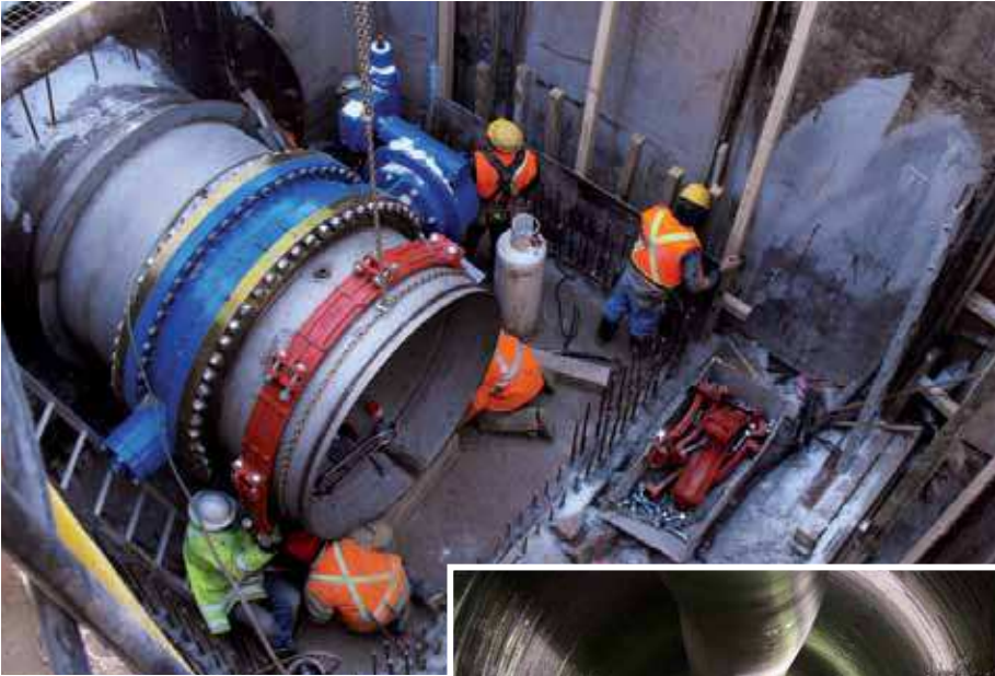
72" (1800mm) Model R-88 couplings used in a domestic water treatment plant, Ontario, Canada
