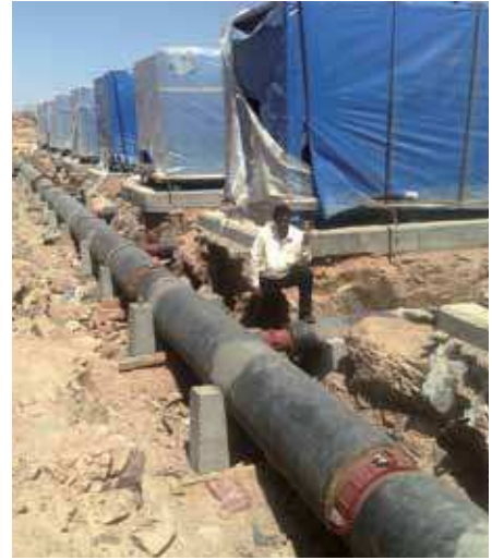
36" (900mm) Model R-88 couplings used in an HVAC chilled water line for a major university, Saudi Arabia
