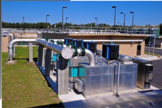
Note: Stainless steel piping is frequently used in water treatment plants because of corrosion resistance and hygienic properties.
